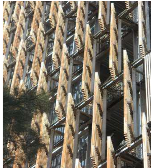
The Shutters on The Western Kinetic Façade System in CH2 Courtesy of the official governmental website of the City of Melbourne, Australia, [Online].
